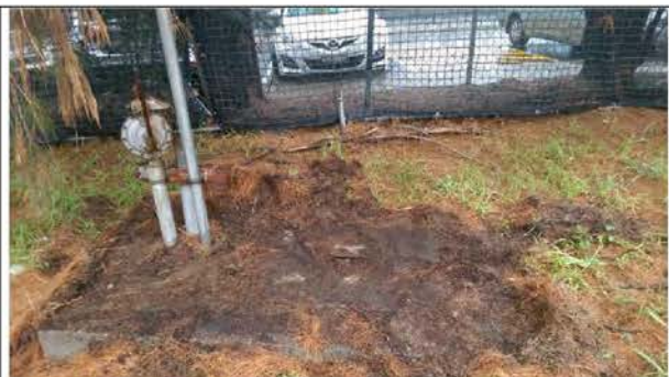
Photo 2: concrete slab with hand pump and vent pipe.
